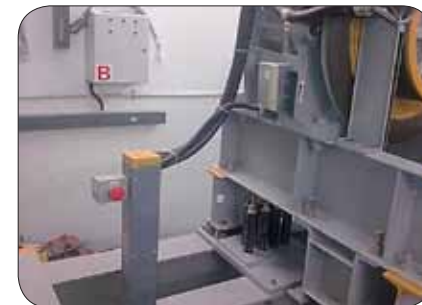
Figure 28: An example of an emergency stop switch next to drive sheave.
