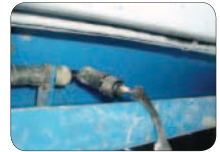
Figure 12: Damaged electrical cords.
