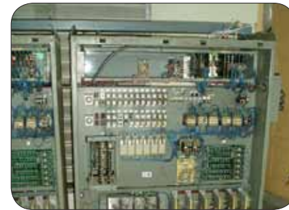
Figure 11: Electrical panels without covers can expose workers to electrical hazards.
