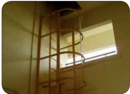
Figure 24: An example of ringed hoops used for the cat ladder near the building opening.
