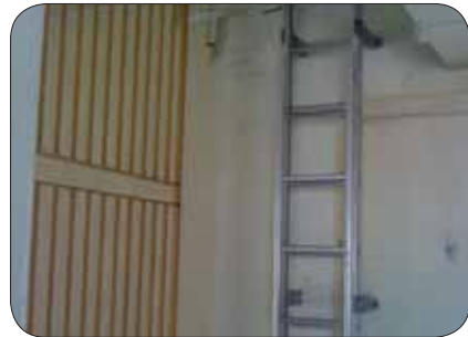
Figure 25: An example of vertical cat ladder in a single plane.
