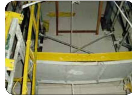
Figure 21: Falling off improperly constructed platform.
