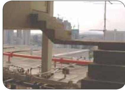
Figure 18: Falling off the edge of the stairs.
