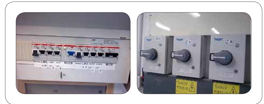
Figure 32: Examples of clear marking on lift isolators and distribution boards.
