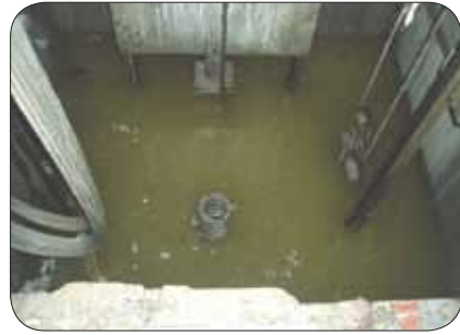
Figure 16: Flooded lift pit.
