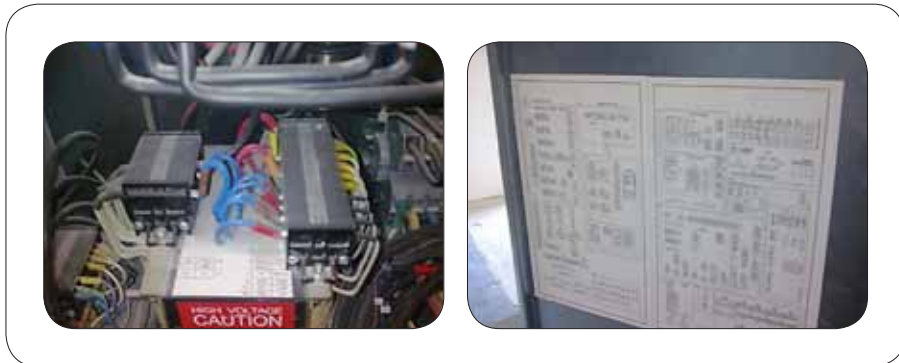
Figure 31: Examples of clear marking and labelling on electrical wires and terminations.
