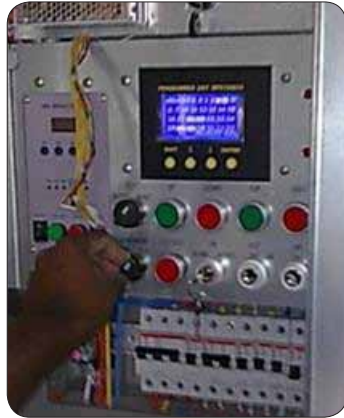
Figure 2: An example of tripping the overspeed governor through a remote device outside the hoist way.
